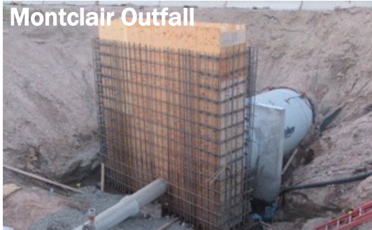
Delgany Wastewater Pipe
